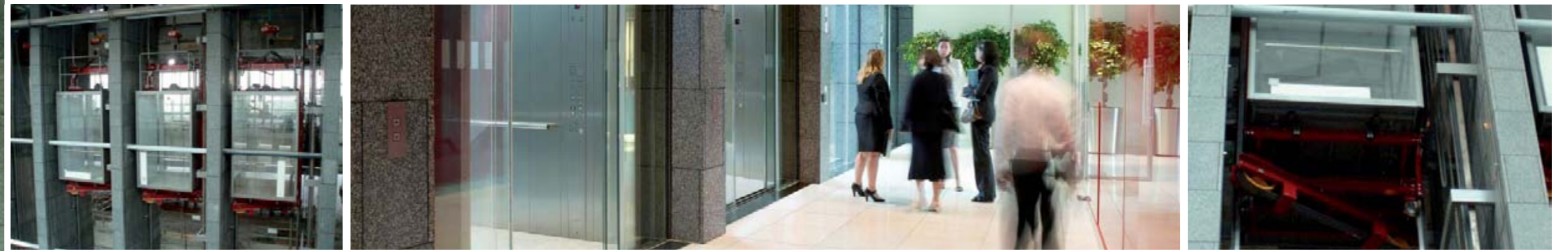
MP GLASS lift Grand Canal Dublin, Ireland Lifts: 4 MP2016G "S" Tailor-made cabins
